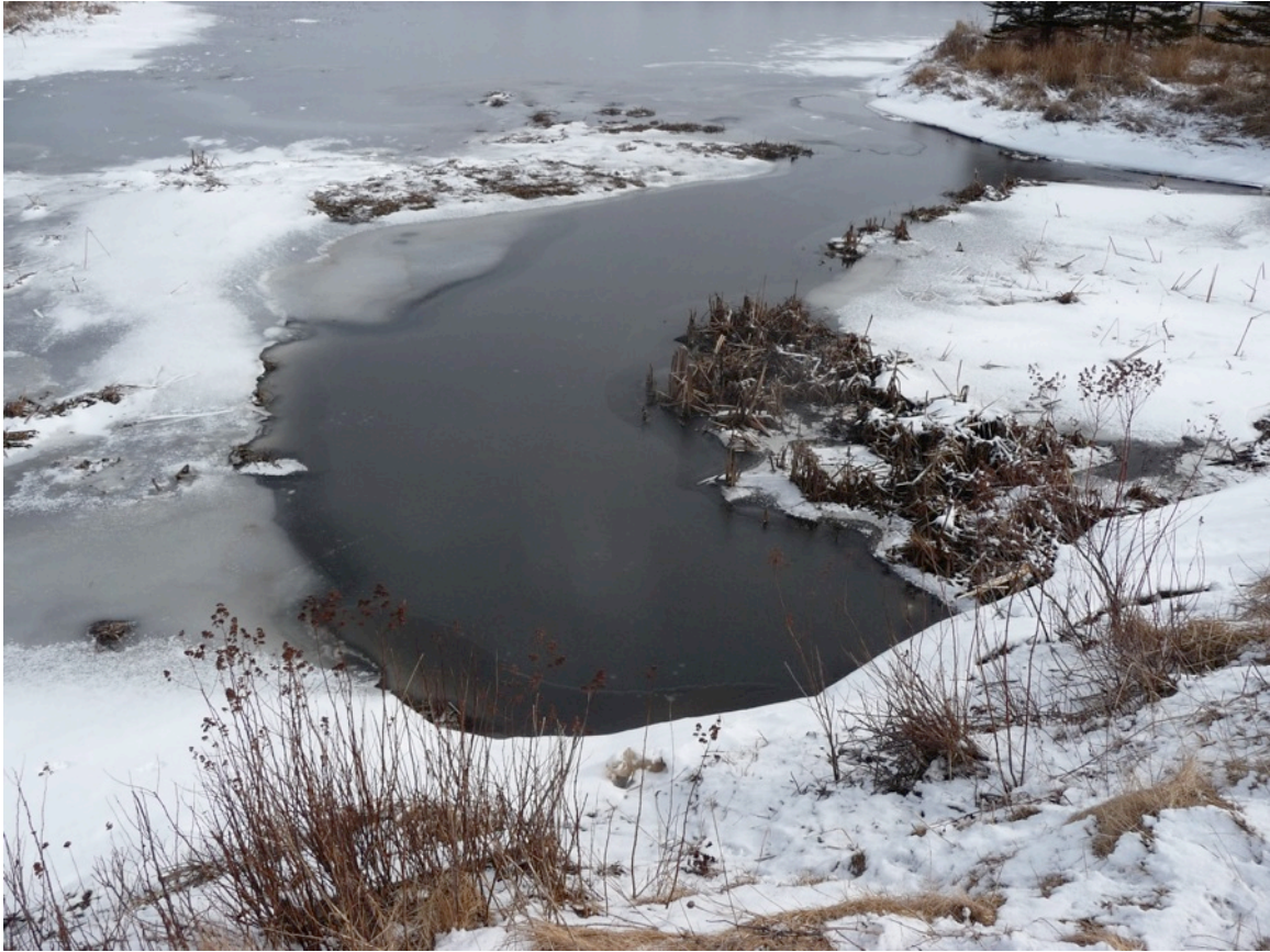
Figure 28 Ice-free channel immediately upstream of the culvert. Photograph by T. Bowron, 6 March 2012.
