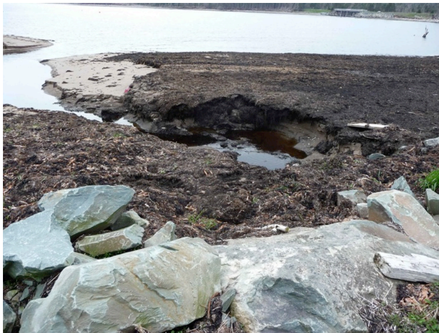
Figure 5 Downstream end of culvert buried by armour stone, and the temporary channel that was created by the spring freshet. Photograph by T. Bowron, 25/6/11.
